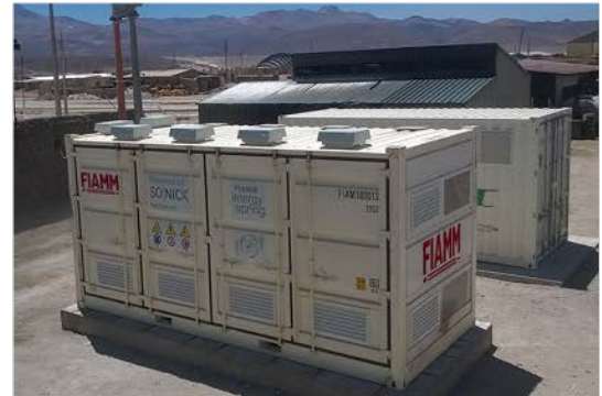
FIAMM (I) storage system: 75 kW/270 kWh http://www.fiamm.com/en/emea/energy-storage/prodotti/spring.-mod-312.aspx
