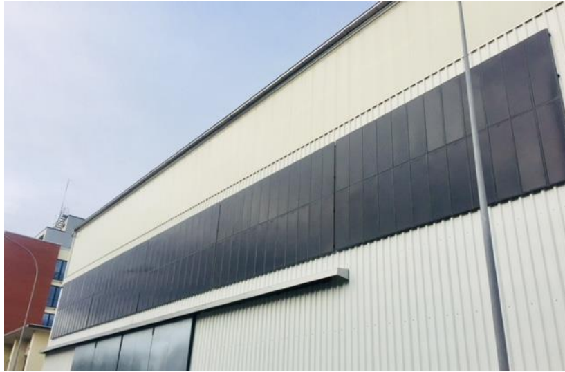
Figure 2.3 Façade BAPV installation with Flisom eMetal modules, laminated on black aluminum
