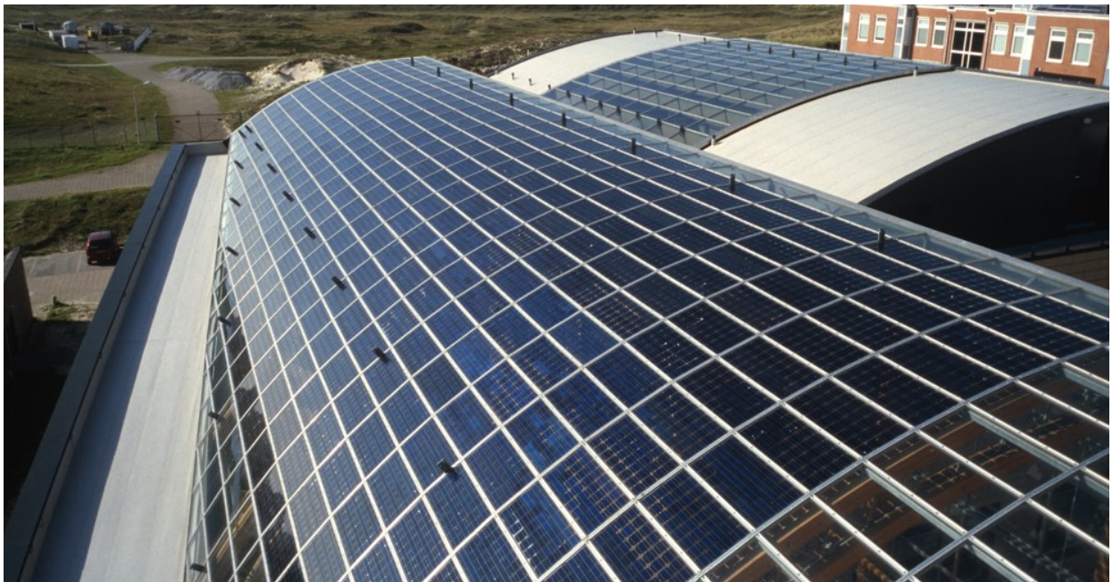
Figure 8.8 Curved roof of the lobby of ECN building 42, Petten. Design: BEAR-iD, Tjerk Reijenga
