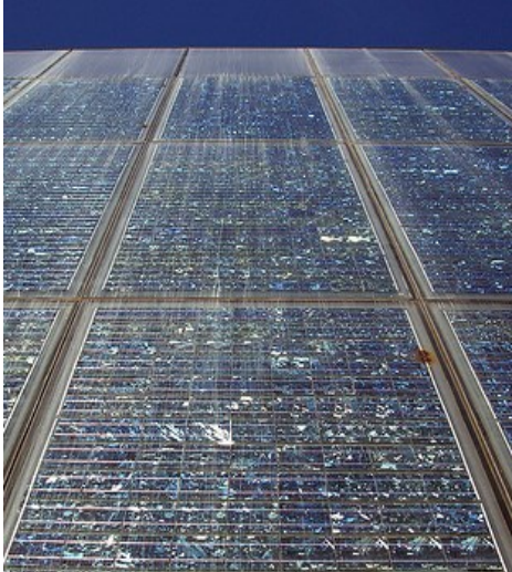
Figure 6.1 Use of non-structural transparent panels in frames. Pompeu Fabra library, Mataro (ES)
