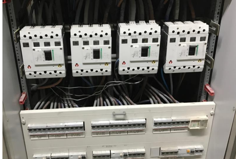
Figure 3.24 Electricity meters installed in the electrical board and covering the consumptions of the offices areas of the building
