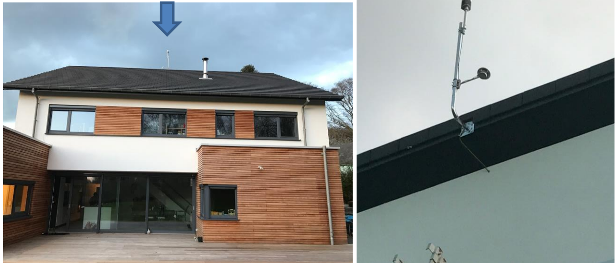
Figure 3.3 Weather station and pyranometer installed on Format D2 house
