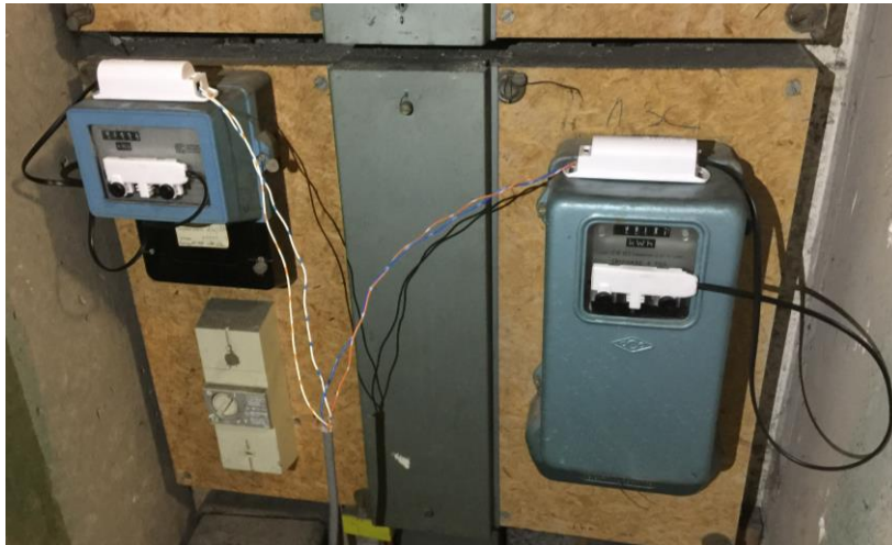
Figure 3.16 Fludia sensors connected on various electricity meters corresponding to lines feeding common spaces of the building
