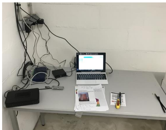
Figure 3.20 Monitoring control room (gateway, computer for remote access...)
