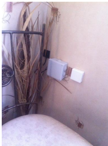
Figure 3.18 Air temperature/relative humidity sensors and wall temperature sensor
