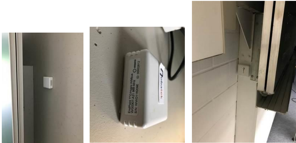
Figure 3.9 Wireless T/RH sensors installed in Pavillon & and Pavillon 2
