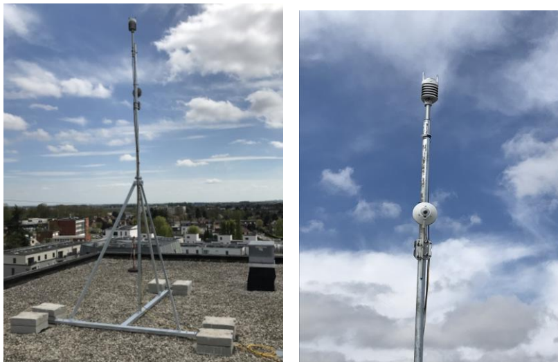
Figure 3.17 Weather station and pyranometer installed on the roof of the building
