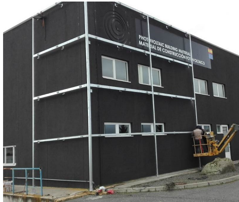
Figure 2.5 S-Vitech PV ventilated façade structural system installed in ONYX’s facilities. Source: ONYX
