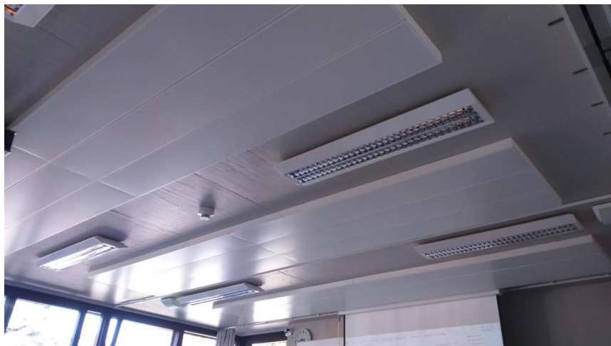
Figure 4.8 Cooling emitters in a classroom of Pavilion 2
