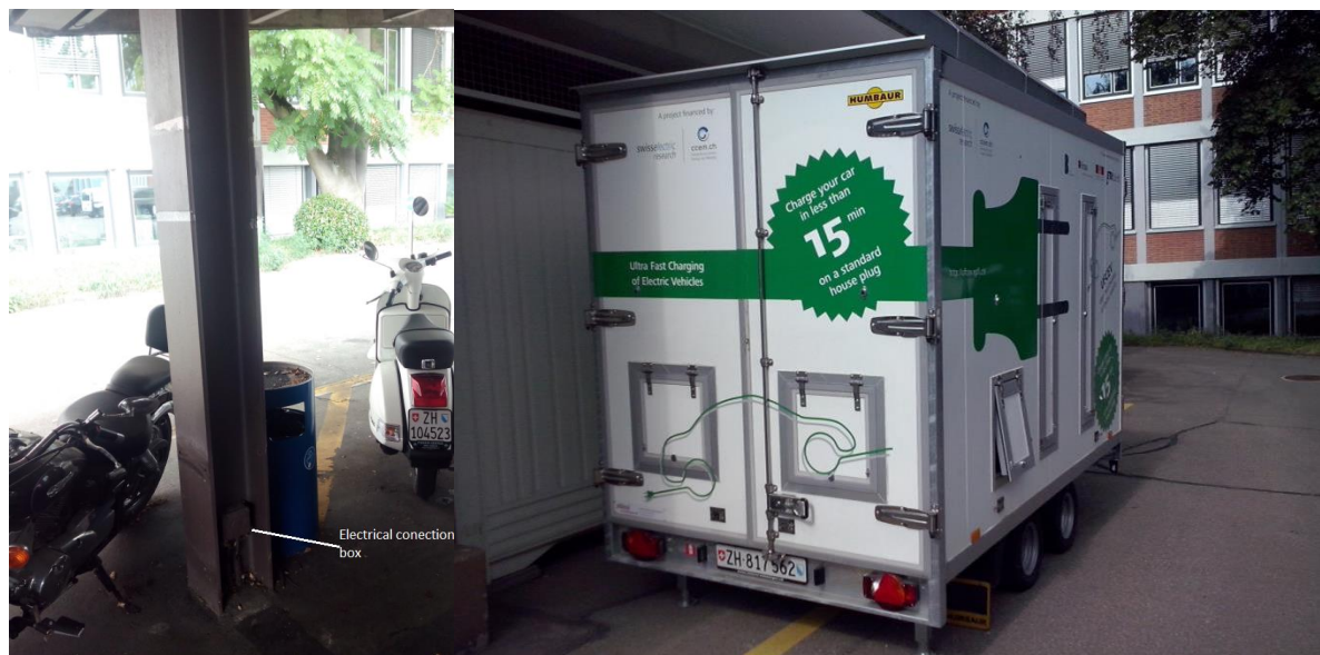
Figure 4.11 Electrical supply box (left) and 20 kW EV charger (right)
